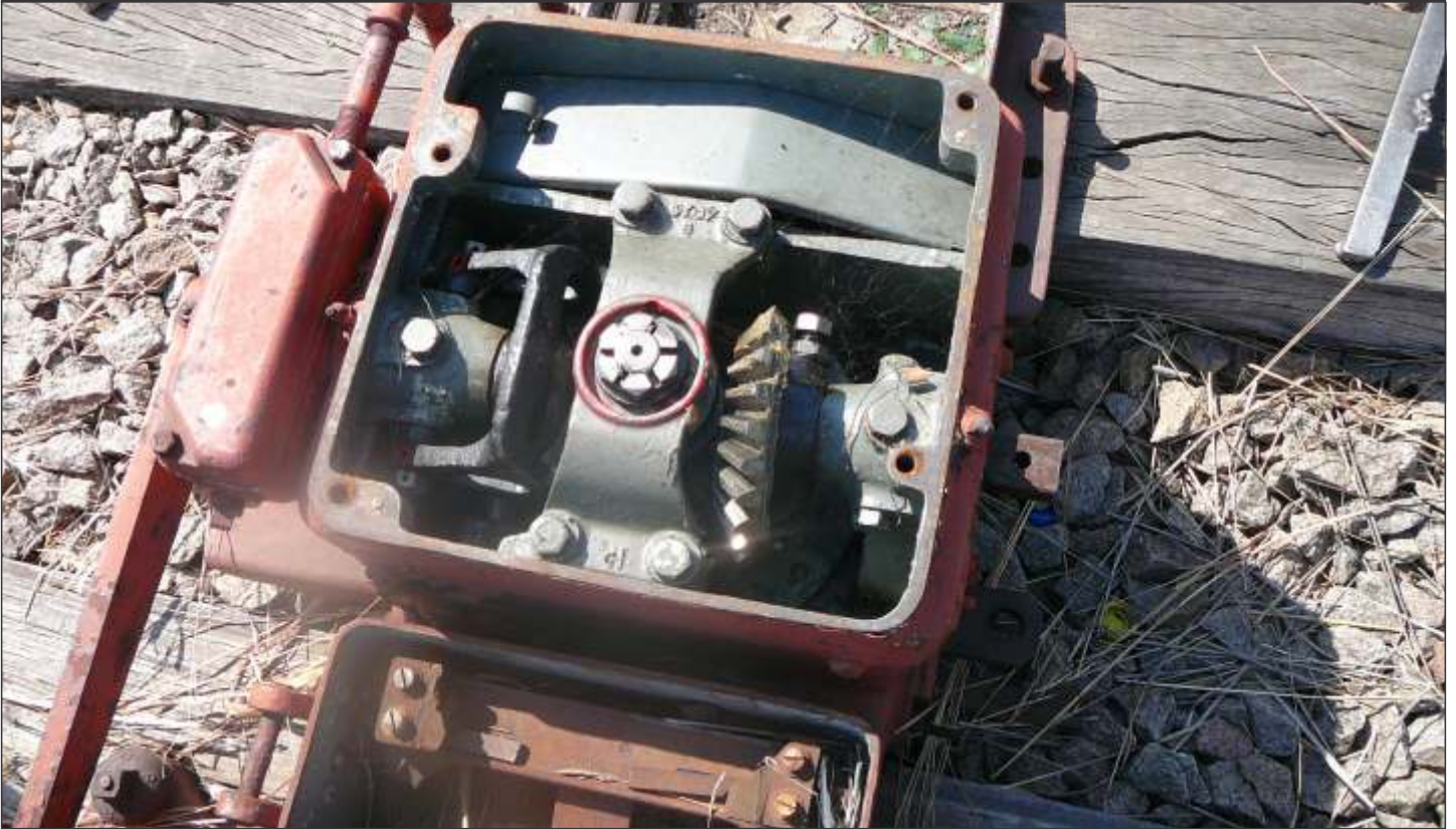
A vandalised points machine where thieves target components
