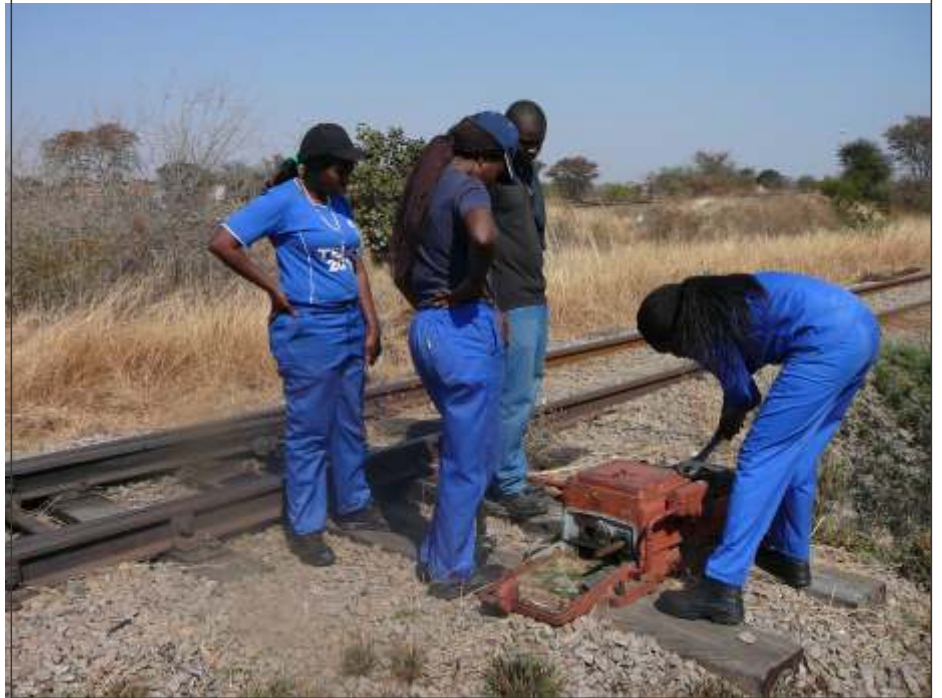
NRZ signal staff check a vandalised points machine in this file picture
