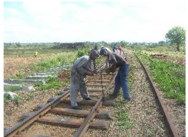
Workers from Civil Tracks rehabilitate a line between Mpopoma and Grain Marketing Board depot in Bulawayo
